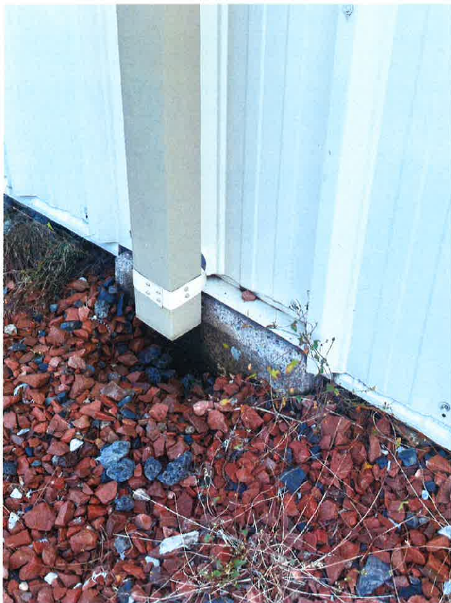
Photo 5: Roof drain discharge directed to building foundation.
