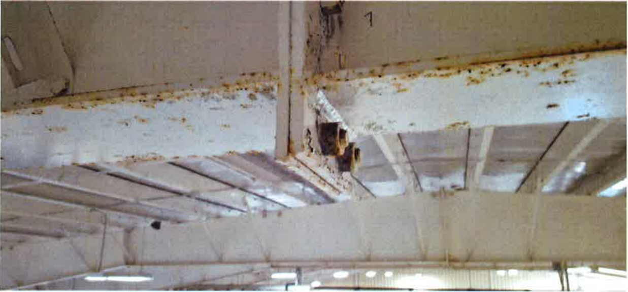
Photo 7: Minor surface rust on bottom flange of building frames. Typical condition.
