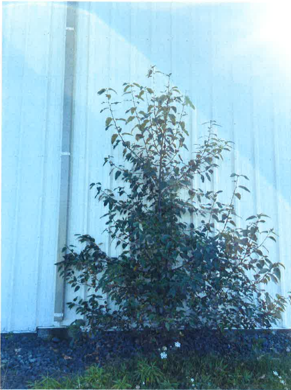
Photo 4: Vegetation growth at building foundation.
