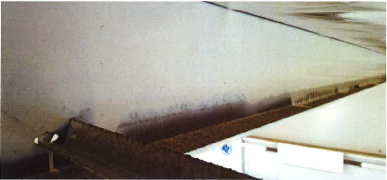
Photo 8: Inconsistent paint coating (exposed primer).
