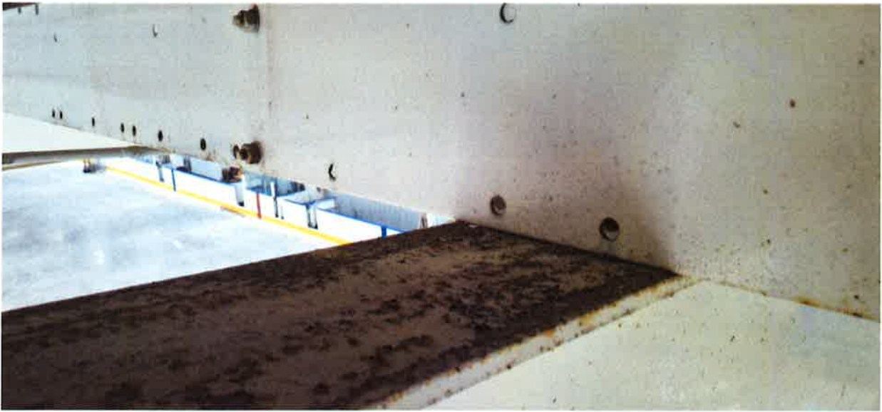
Photo 7: Minor surface rust on top of building frames. Typical condition.
