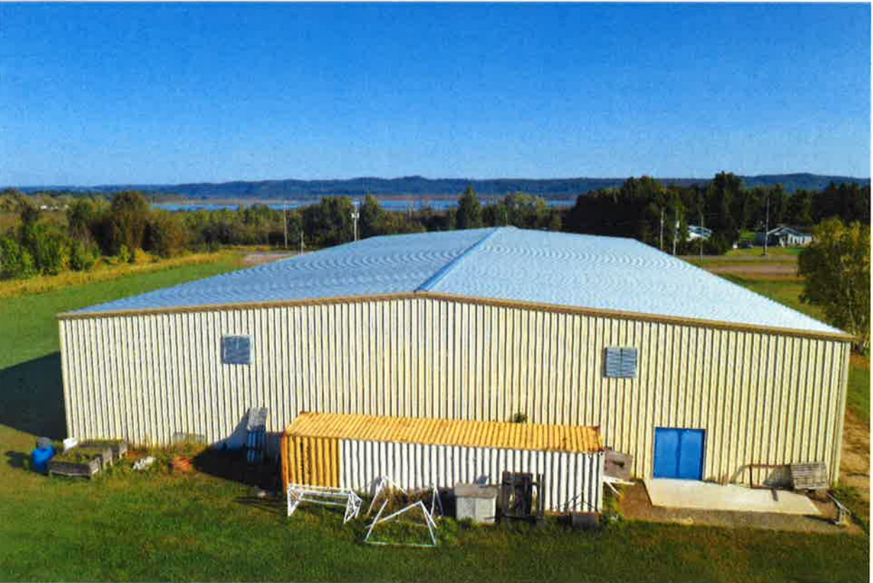
Photo 2: View of south end of arena building. Note 2 ventilation fans no longer in-use.
