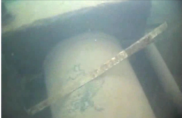
Photograph 7: Loose stainless steel casing strap
