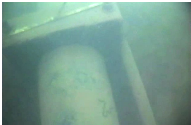
Photograph 5: Chlorine line conduit strapped to ballast
