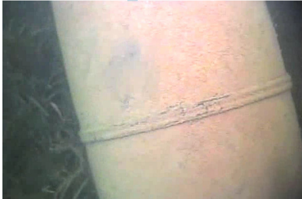
Photograph 3: Fused HDPE intake pipe
