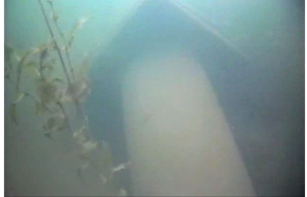
Photograph 8: Crooked concrete pipe ballast
