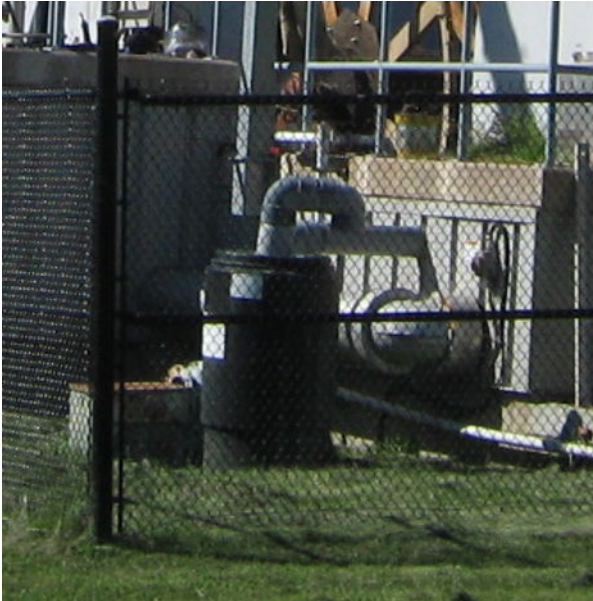
Photograph 8.4: Odour Control Unit #2
