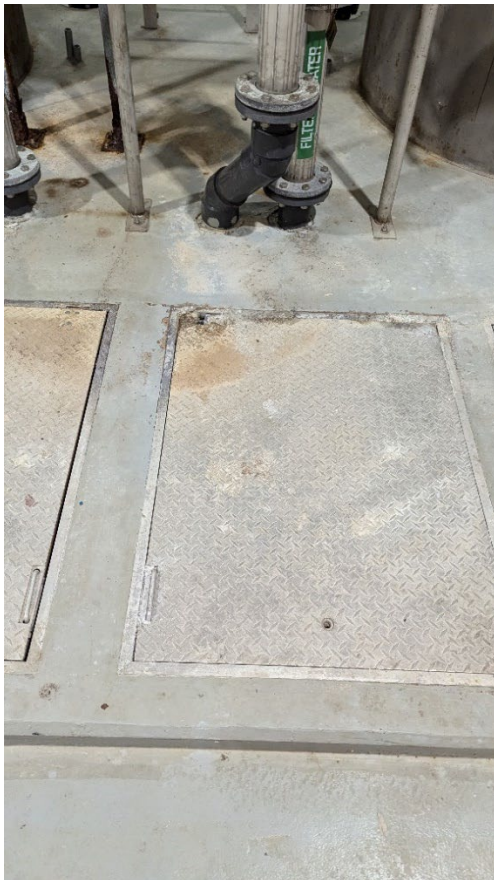
Photograph 7.3: Damaged GAC Well Hatch
