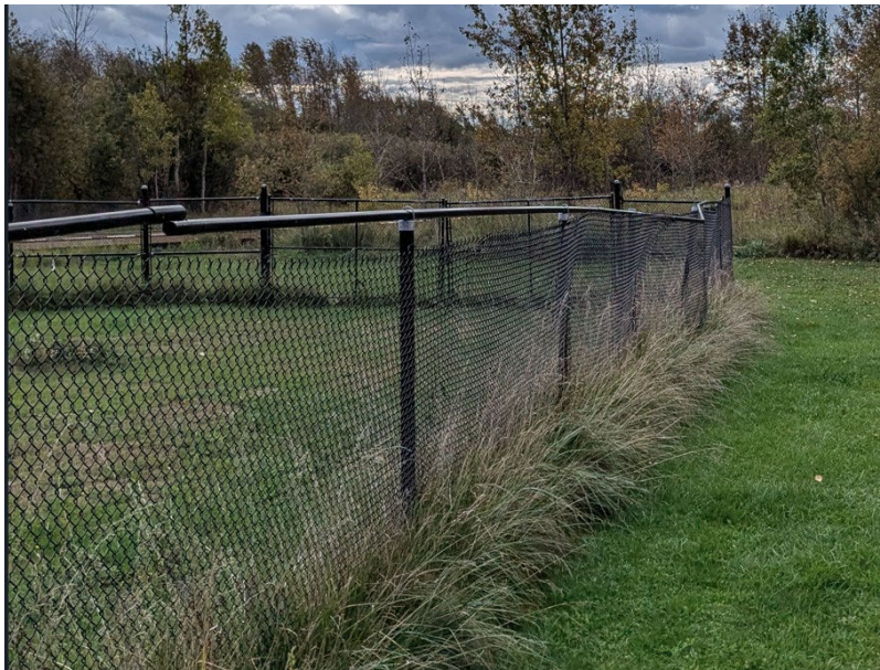
Photograph 7.1: Damage to Chain Link Fence
