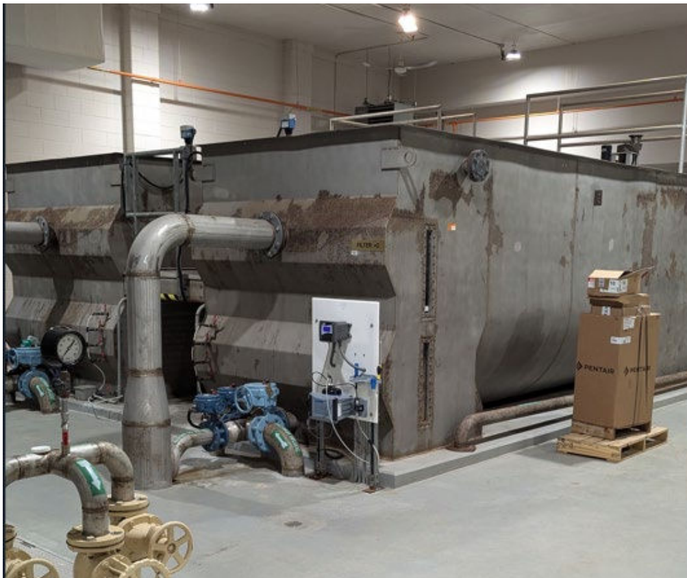
Photograph 7.1: Corrosion on Filter Train Tanks
