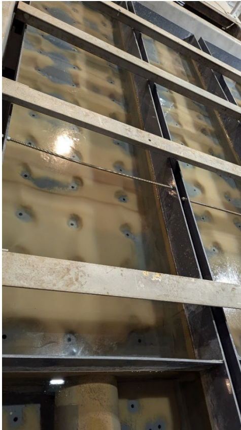
Photograph 7.2: Floc Build-Up on Top of Clarifier Troughs
