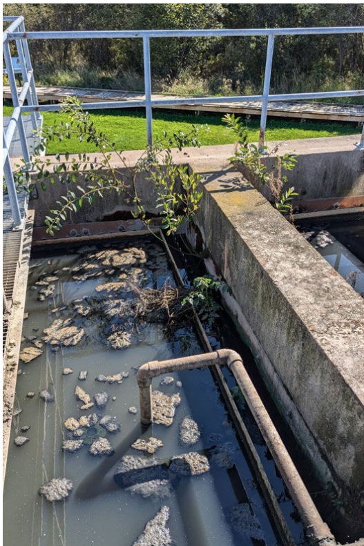
Photograph 8.1: Primary Clarifier Vegetation and Scum Build-Up
