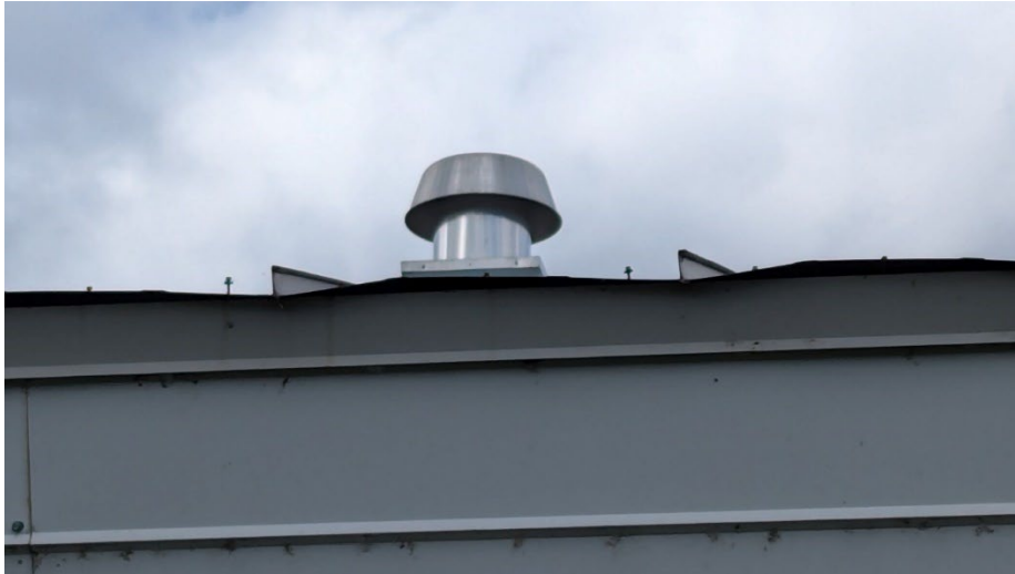
Photograph 7.2: Screws Along the East Roof Edge Requiring Re-Setting
